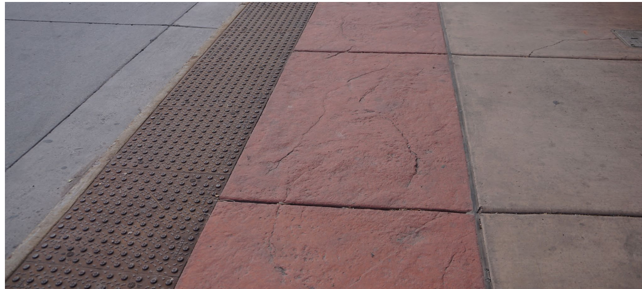
Figure 32: Ground Mounted Tactile Strip
