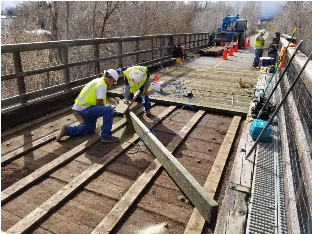
DECK RESURFACING ON THE ROARING FORK BRIDGE ON THE RIO GRANDE TRAIL
