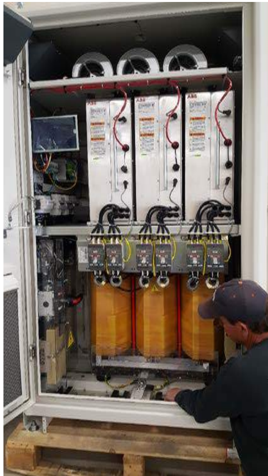
BATTERY ELECTRIC BUS CHARGING INSTALLATION
