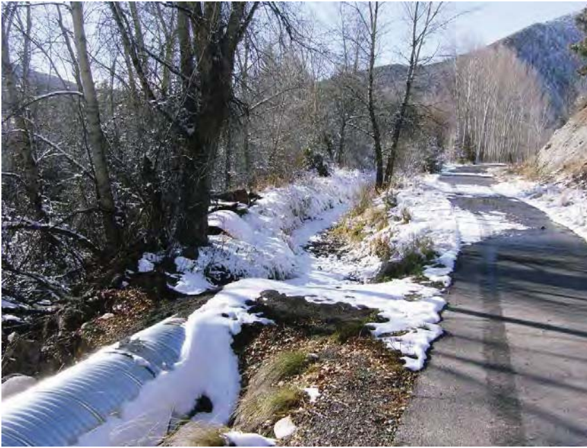
View of new culvert and ditch to left; old culvert parts lie beyond the big tree on the berm to left of ditch.
