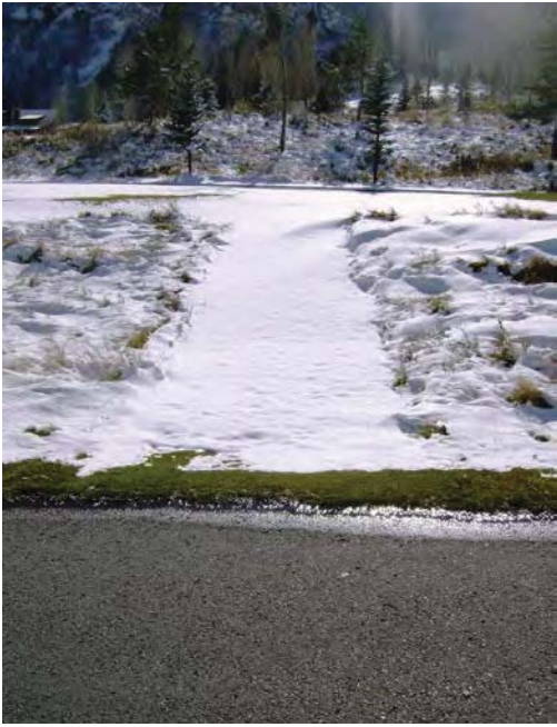
View of path constructed at Roaring Fork Club across trail from staircase
